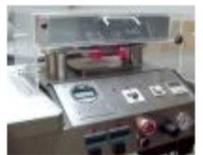
Press Control panel
